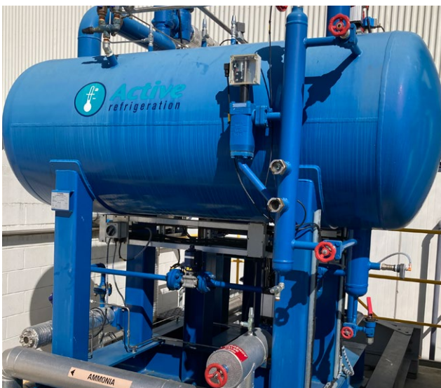
Industry-first High Temperature Industrial Heat Pump at our Nelson site.
